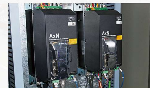
进口电器元件 Imported electrical components
